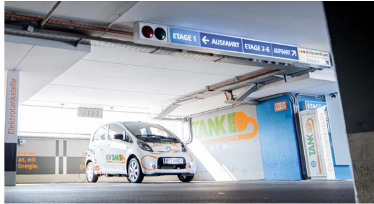
With around 200 charging points, WIPARK car parks are supporting sustainable mobility.
